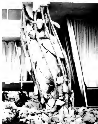
Photo 25. Tied reinforced concrete column having little remaining strength. Ties broke, and the vertical steel broke as shown in photo 26.
